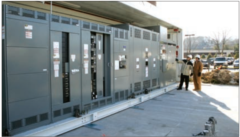
Housing with outdoor switchgear installed at Pall's corporate headquarters is inspected before the other half is set in place.
