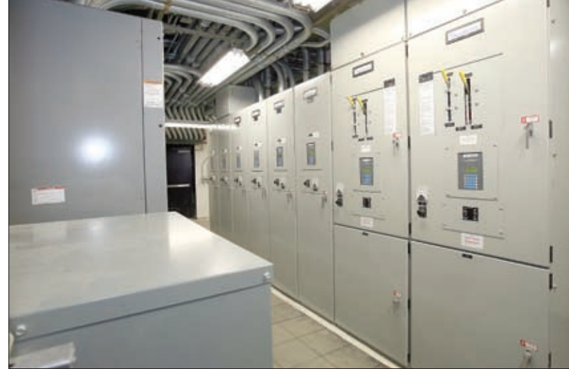
(l.) North Shore University Hospital's emergency power upgrade was installed without any loss or interruption of power. (far l.) Some of Roland's retail clients across the island.
